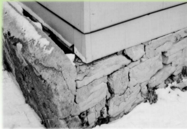
Major Damage to a Foundation Wall
